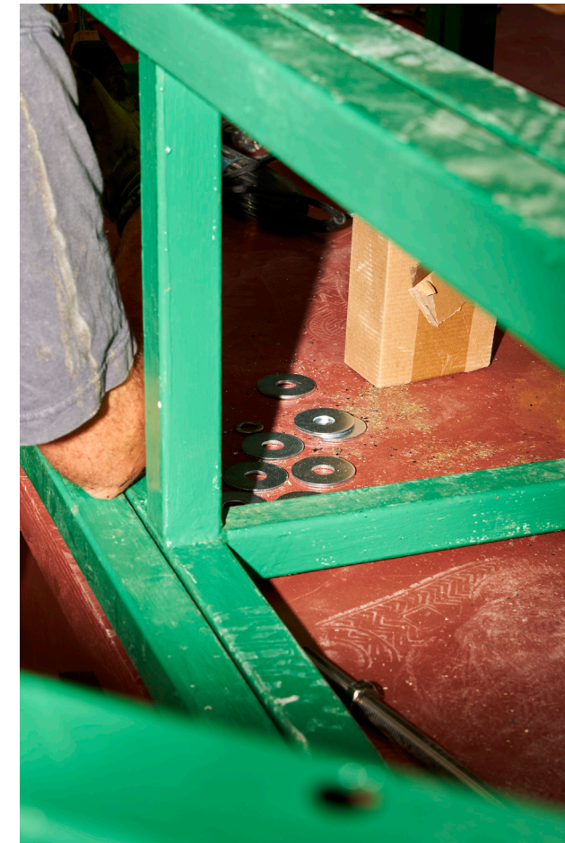
FIG 06. Elementos metálicos reutilizados, lijados y pintados con varias capas, fueron empleados para la estructura principal / Reused metal elements, sanded and painted with several layers, were used for the main structure [Fotografía / Photography Clelia Cadamuro].
